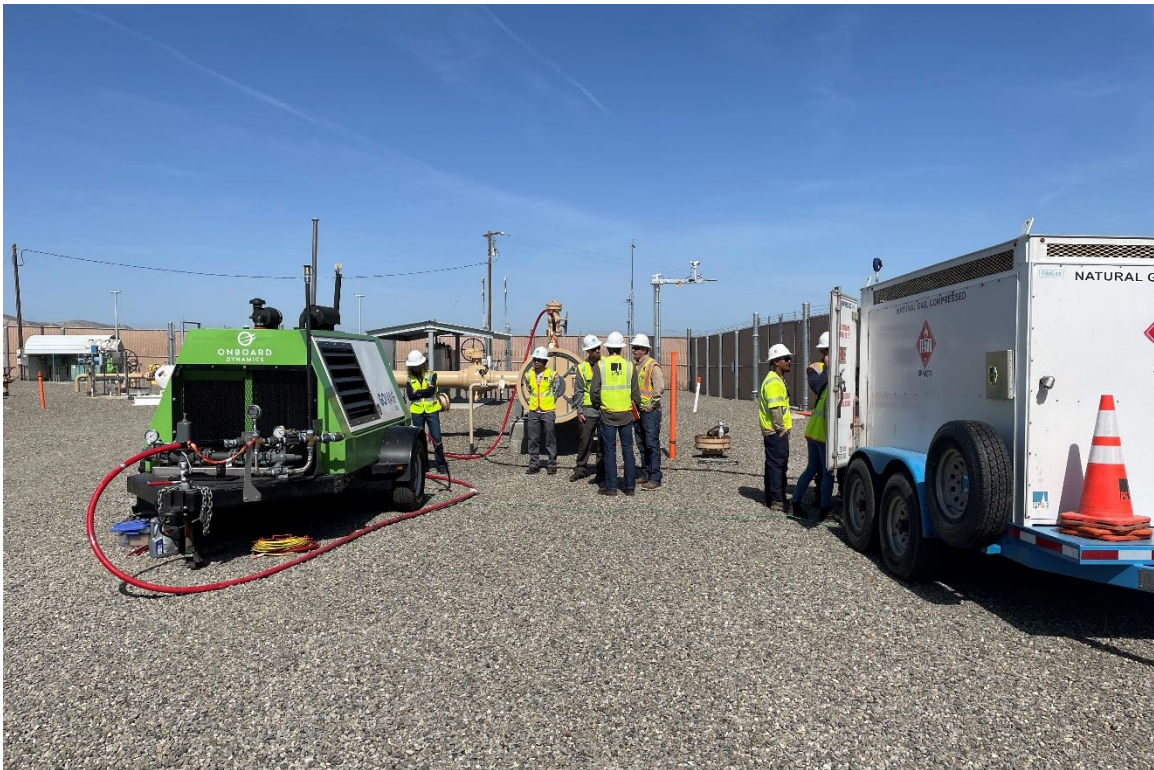
Figure 13. PG&E pig launcher evacuation into a high-pressure tube trailer.
